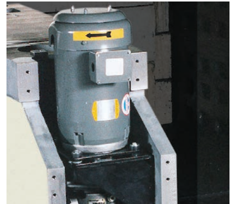
Hydraulic motor pump assembly mounted in left hand rear press bed leg.
