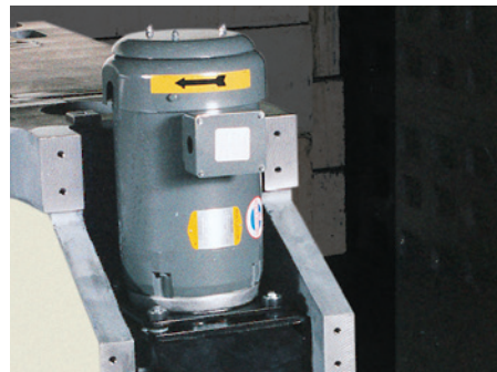
Hydraulic motor pump assembly mounted in left hand rear press bed leg.
